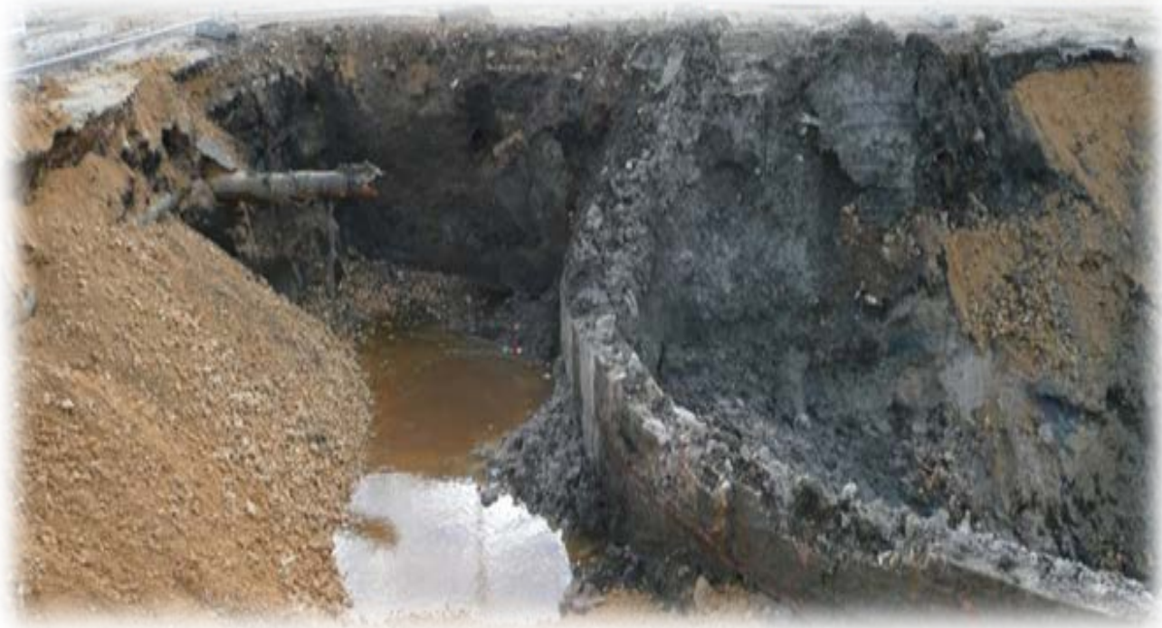
Coal Tar Contaminated Soil at Old Gasworks
