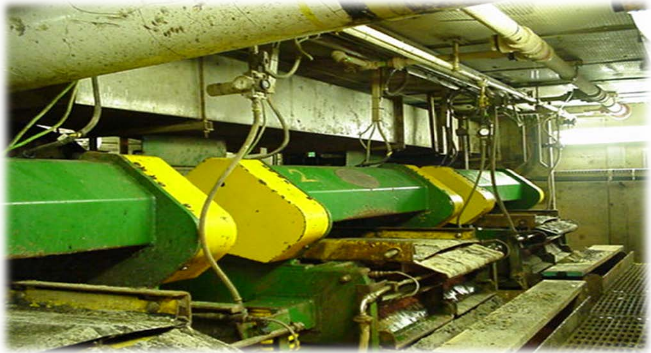
Cuttings Shaker House
